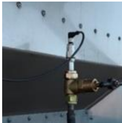
Pressure transducer installed
