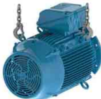
Figure 4.19 - Final result: motor placed in horizontal position
