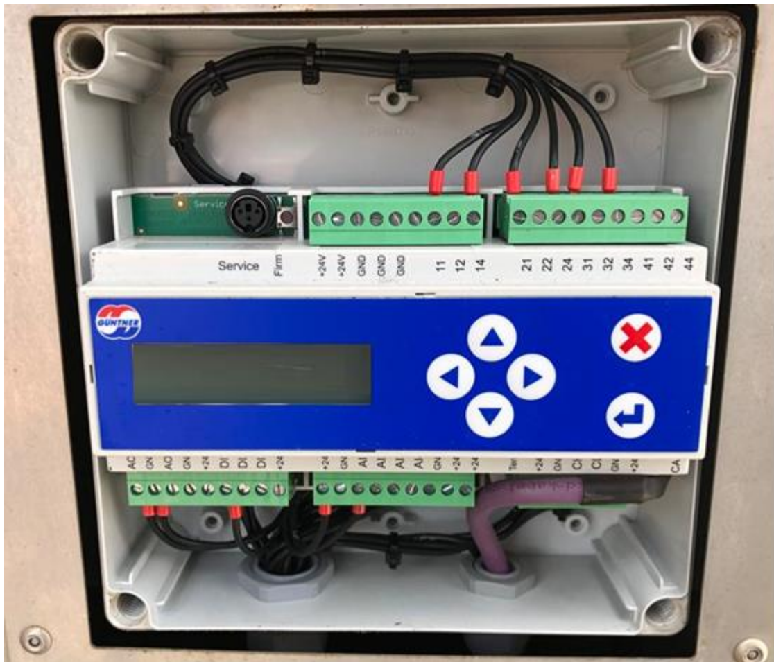
Figure 1: Externally located GMM EC display.
